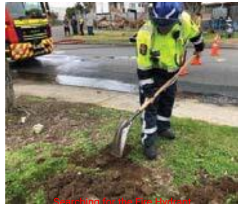
Searching for the Fire Hydrant
